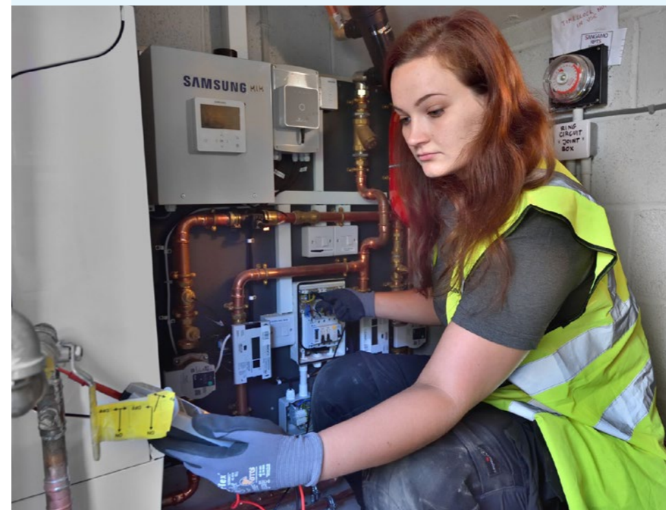
↖ Compliance checks in the plant room for hybrid heat (gas and air source heat pump) in Newtongrange, Midlothian.
